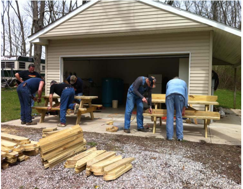
A talented crew - Campground Chairman Mark Drake along with a small group of new members spent clean-up weekend building several new picnic tables. The new tables will be put into service in the Campground and around the lakes. Old and rickety picnic tables were taken out of service. (Greene County Fish & Game Photo by Mark Drake.)
